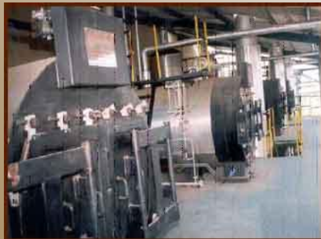
WHRB Installed on Natural Gas Fired Engine
