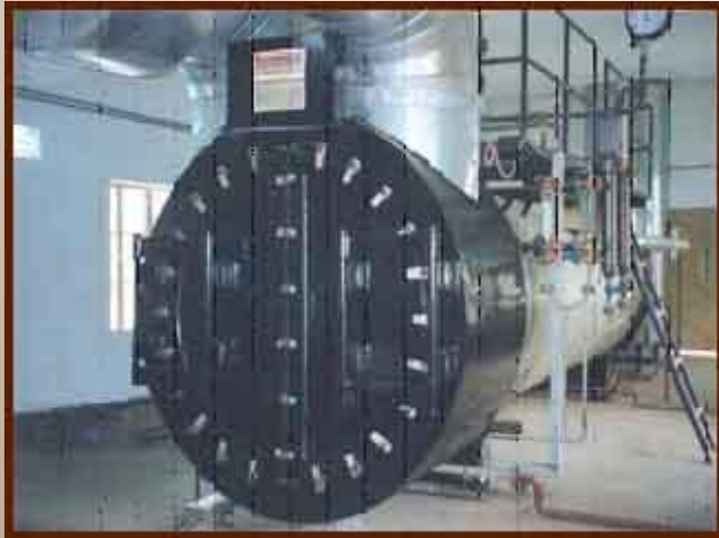
WHRB Installed on Natural Gas Fired Engine,
