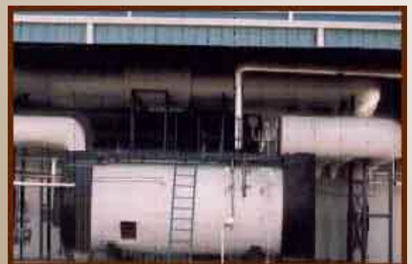
WHRB Installed on Heavy Fuel Oil fired engine
